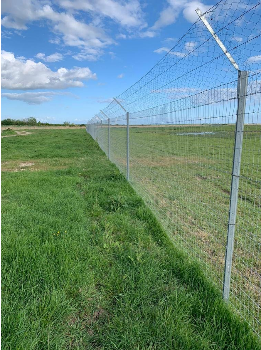
Plate 1. Example of fence installation with the same specification as that to be installed at AOE SPA. Note that the vegetation along the outside edge has fully recovered following replacement over the buried skirt.
